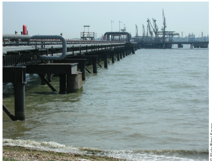
Hamble Oil Terminal, UK.
